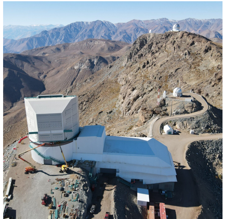
The Rubin Observatory, which will take nearly a decade to complete, has a unique appearance compared to other observatories due to its large support building that will act as a maintenance shop for the supersized camera and telescope. (Rubin Observatory/NOIRLab/NSF/AURA)
